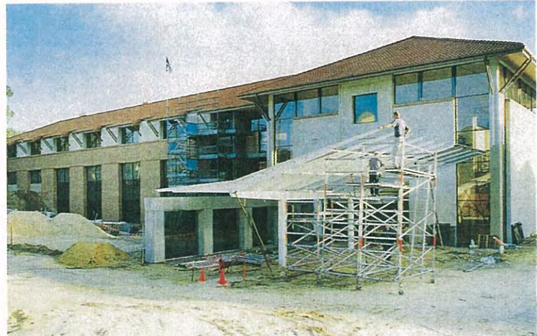
The new 120 bed ward block under construction at Hollywood Private Hospital. The ward is expected to open in August 1997.
